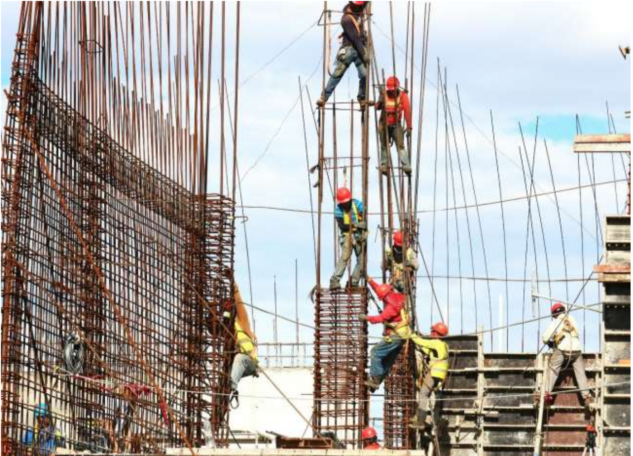
This image from Costa Rica demonstrates how the common construction process of building upward floor by floor means workers responsible for the preparation for concreting (rebar and form work) are always exposed to the sun. Photo by Josue Isai Ramos Figueroa, 2018. Unsplash . Public domain .
